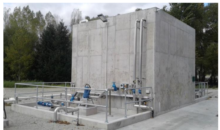
Figure 8: Septage reception system (mixing and transfer pumping system visible)
