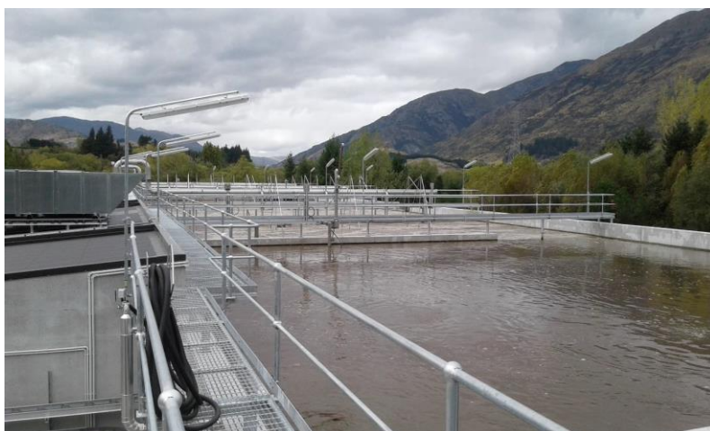
Figure 4: View across MLE reactor (Anoxic Zone 4 in foreground)
