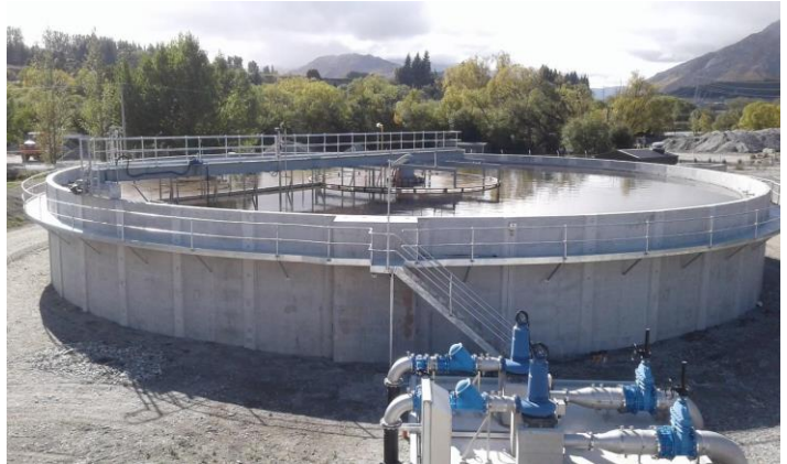
Figure 5: Clarifier tank (RAS pumps in foreground)
