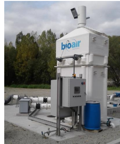
Figure 7: Odour treatment system
