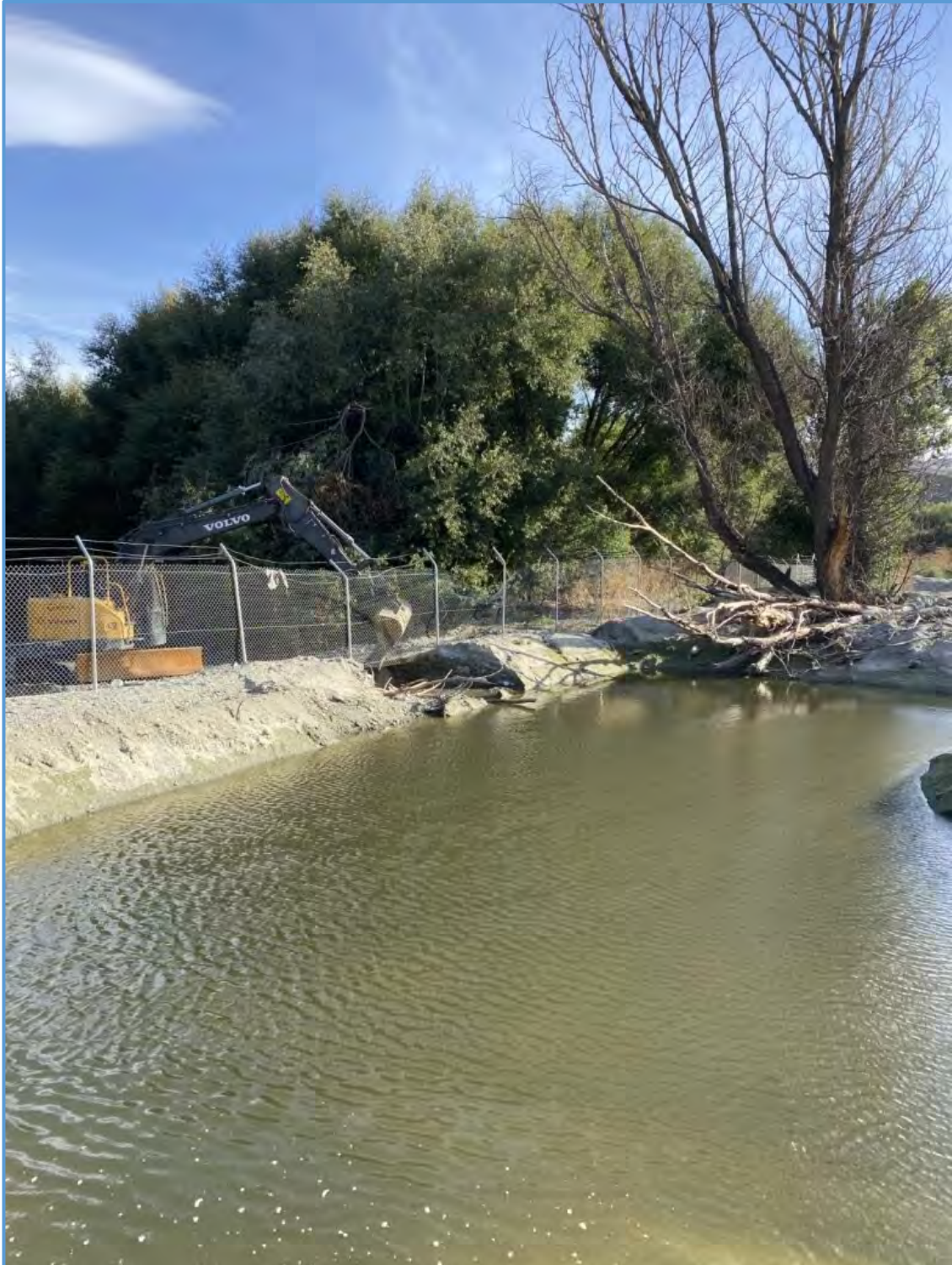
Figure 24: Showing earth bund breach from Disposal Field under South boundary fence.
