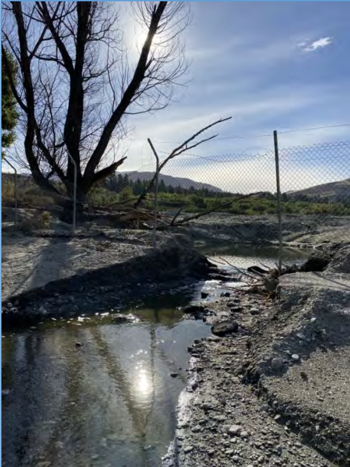
Figure 25: Earth Bund breach under the South Boundary fence.
